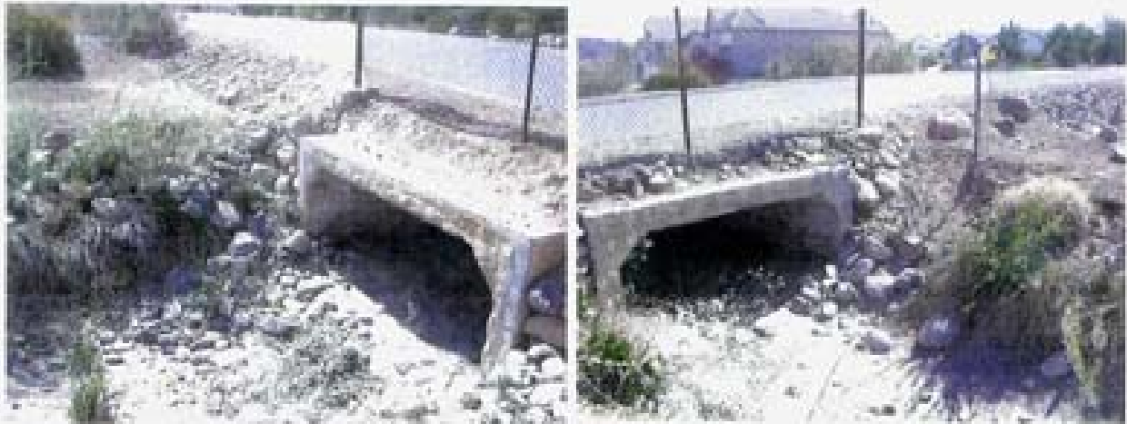
Point 47. Box culvert conveying flow under Wolf Run Lane. Note the small swales draining into the ditch.
