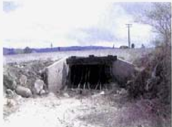
Point 53. Box culvert conveying the Steamboat Ditch under the Mt. Rose Highway. A large amount of fine sediments and trash have accumulated in this section of the ditch.
