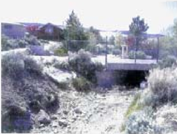
Point 28. Box culvert under Odile Ct. A shallow, concrete swale drains stormwater from the road into the Steamboat Ditch.
