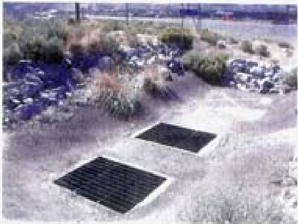
Point 54. Stormwater runoff flowing off the Mt. Rose Highway enters the Ditch through these grates.
