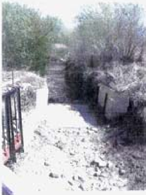
Point 48 cont. Weir structure and sluice gates adjacent to Arrow Creek Parkway.
