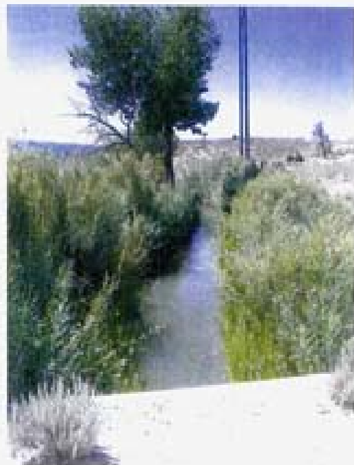
Point 57. Outlet of the box culvert downstream of the Mt. Rose Highway and adjacent to the powerplant.
